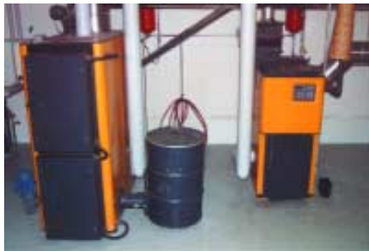
Two wood pellet boilers, used to heat a school in Denmark
