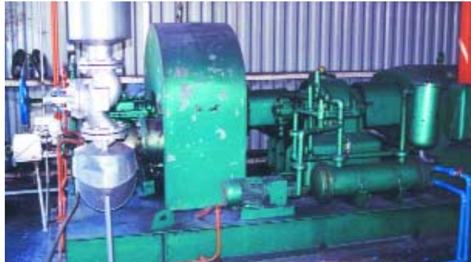
Example of a small-scale biomass fired CHP system. In a rice drying and packaging plant in Malaysia, rice husk is burned in a water cooled step grate furnace to generate steam (17.5 Bar) for a single stage 225 kW e backpressure turbine. Remaining heat is used for paddy drying. (Courtesy of TNO, The Netherlands)
