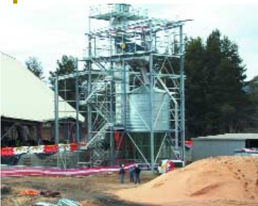
A biomass fuel handling facility which directly meters biomass onto the coal conveyor belts at the Wallerawang Power Station, Australia (Courtesy of Delta Electricity, Australia).
